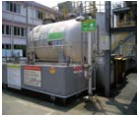
Hazardous chemical storage tank
