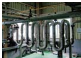
Chemical mixing devices in the water quality treatment facility
