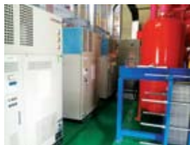
Heating pumps that recycle waste heat
